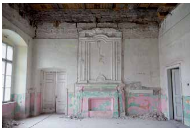
Fig. 4 Photo of the lime mortar chimneypiece in the room II. Test windows in the chimneypiece with well preserved fragments of the decoration. Phot. W. Holnicki
